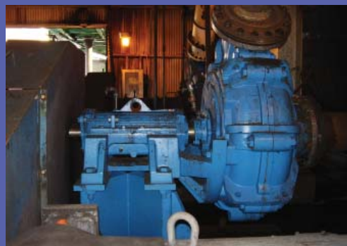
Heavy Media Cyclone in a Coal Preparation Plant
